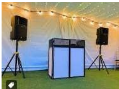
Lighting and sound equipment
