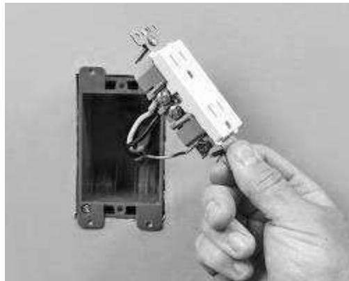
Installed wall socket
