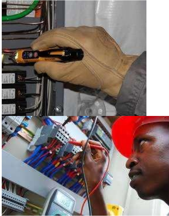
Person testing a electrical circuit
