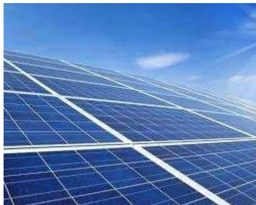
Solar power plant
