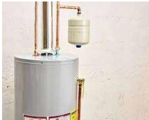
installed water heater
