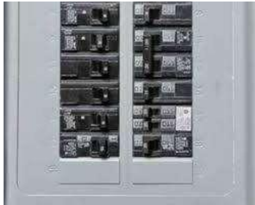
Circuit breaker panel
