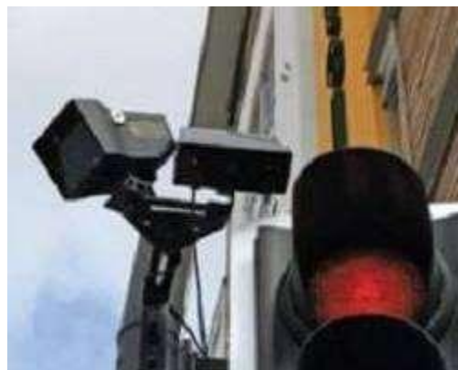
Pedestrian crossing sensor
