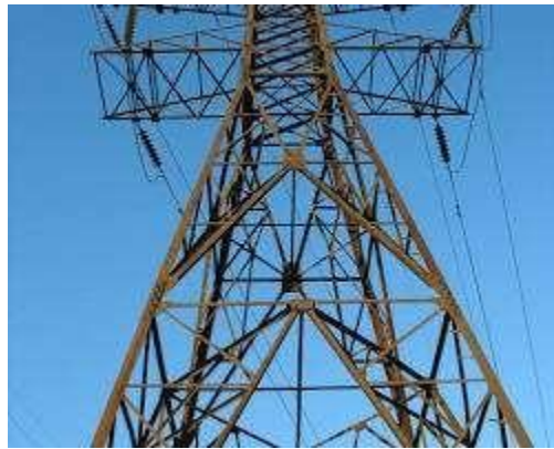
high voltage transmission towers
